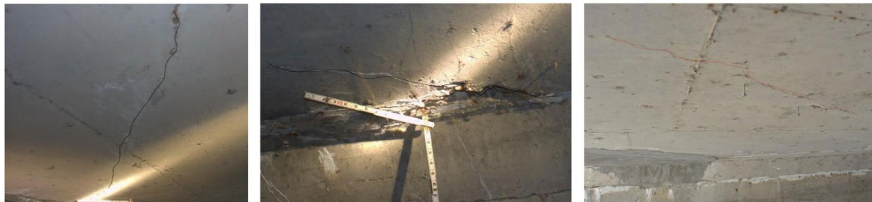
Fig. 2. Cracks underneath concrete bridges (Andrawes et al., 2024).
