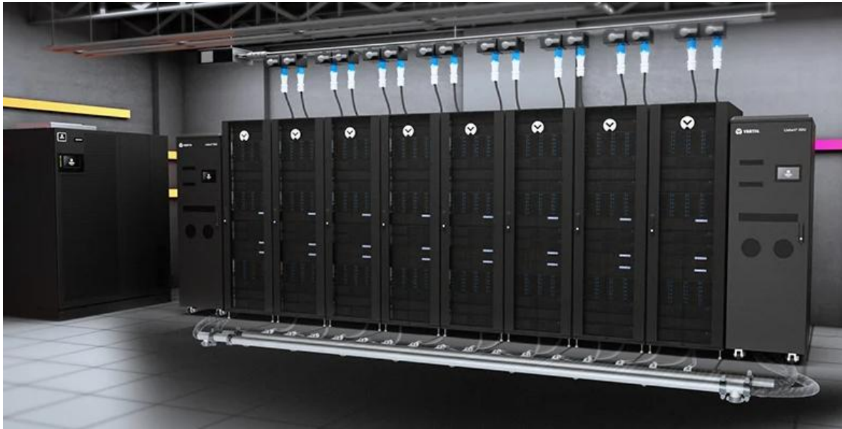
Technical Water to CDU (Coolant Distribution Unit)
