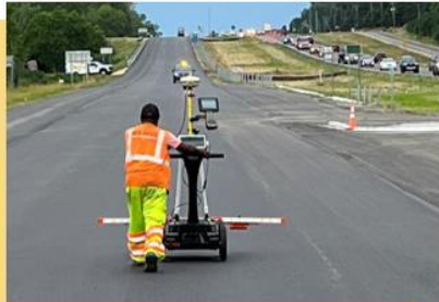
By rolling a DPS unit over the newly paved roadway, crews measured the pavement's density in real time.
