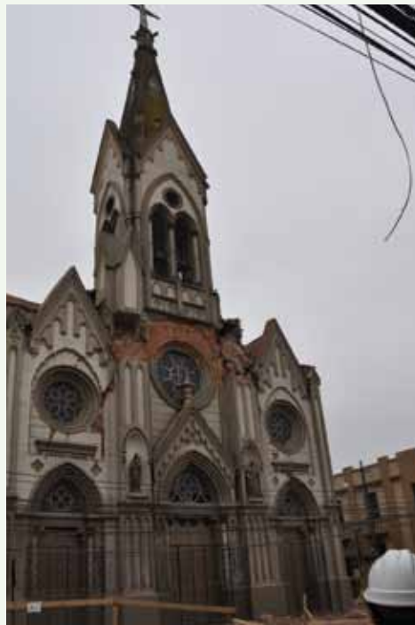
◀ Damage at the Campanario Iglesia Salesiana de Talca in Chile.
