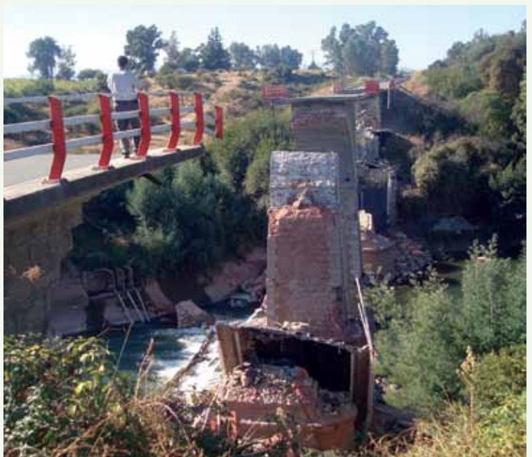
A member of the GEER team examines a failed bridge in Chile.
