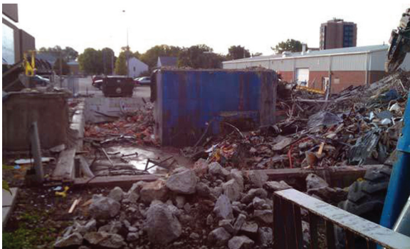
Remains of the TRIGA reactor bioshield. The project was completed and the area was cleared over the summer.
