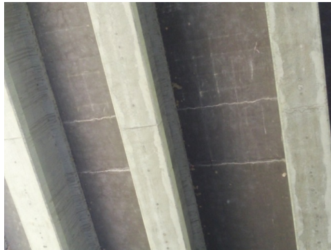
A. Transverse cracking in a concrete bridge
