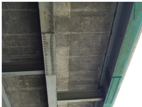
B. Transverse cracking in a steel girder bridge
