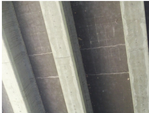
A. Transverse cracking in a concrete bridge.
