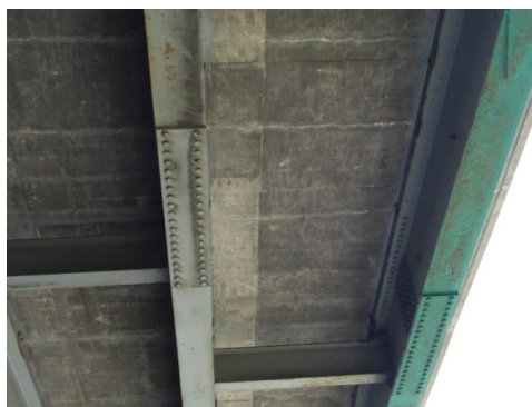
B. Transverse cracking in a steel girder bridge.
