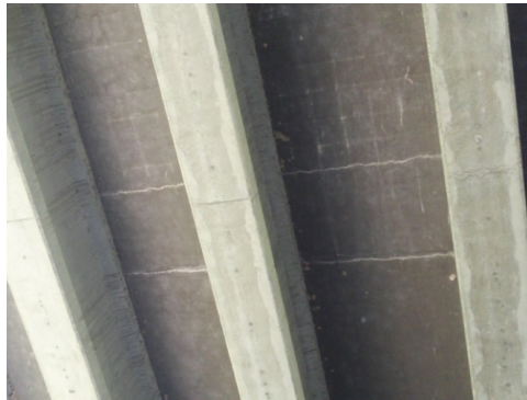
A. Transverse cracking in a concrete bridge.
