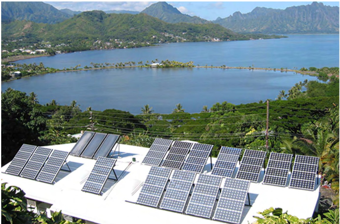
Figure 2.3 A 4 kW GPV system in Kaneohe, O'ahu, Hawai'i
