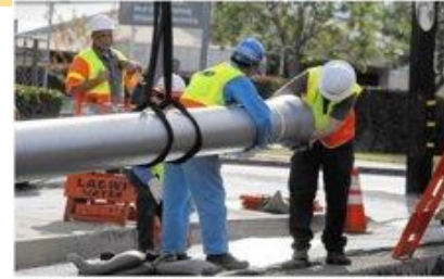
U.S. Department of Water and Power workers install an earthquake-resistant water pipe in Northridge in January. 2007 engineers schedule it will cost $35 billion to reinforce water pipes throughout the city. (Gary Friedman / Los Angeles Times)
