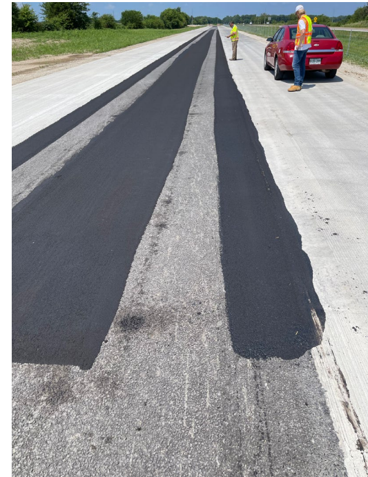
Artificial Rutting Section
