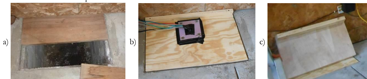
Figure 2 Images of the various crawlspace access hatches at site 4: a) the original hatch with one plank set aside, b) a more air-tight temporary hatch with a pass-through for sample and pressure tubing, c) the permanent hatch
