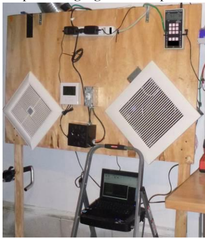
Figure 3 The temporary fan apparatus installed in garages
