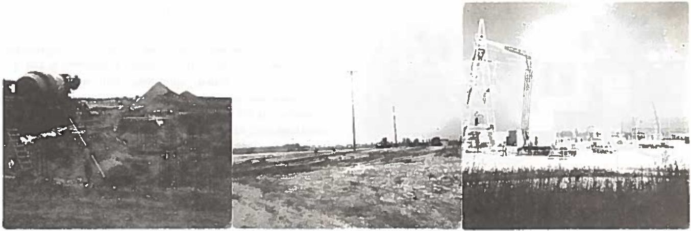
COMMONWEALTH EDISON'S ELECTRICAL SUBSTATION CONSTRUCTION. Left: rough-graded site with temporary electrical supply and construction trailers. Center: Installation of foundations. Right: stringing of wires to a transformer in the 138,000 volt yard in the foreground.
