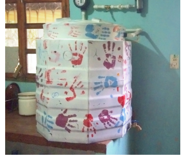
Mary Beth's parents photographed the still-operational clean water system during a return trip in November.
