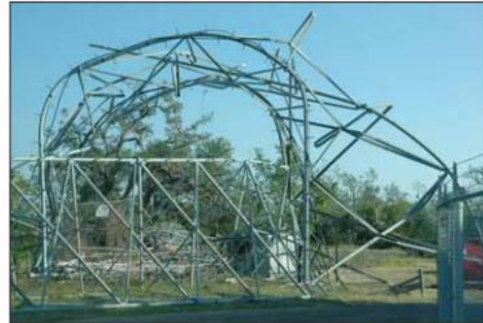
A downed communications tower, Plaquemines Parish, LA.
