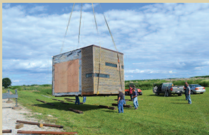
The Element House was transported on three trucks from Chicago to Urbana in August 2013.
