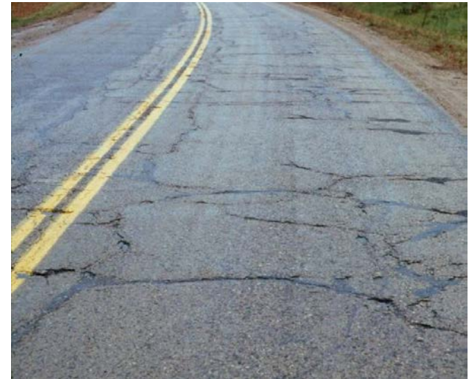
Block Cracking (All HMA)
