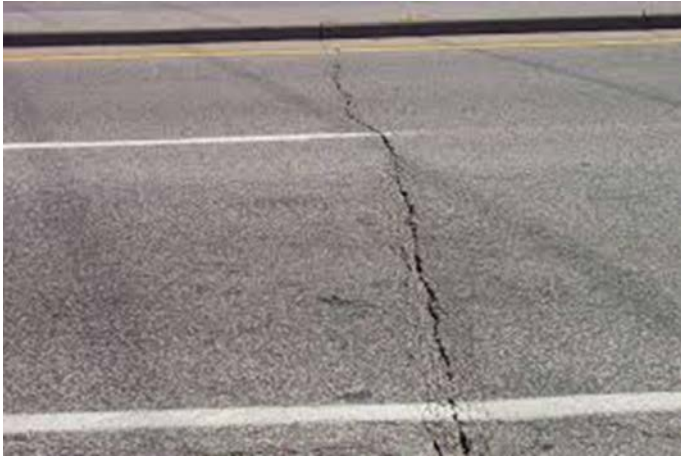
Thermal Cracking (Full Depth HMA)
