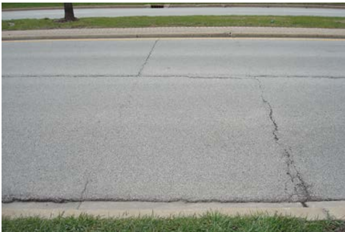
Reflective Cracking (Composite)
