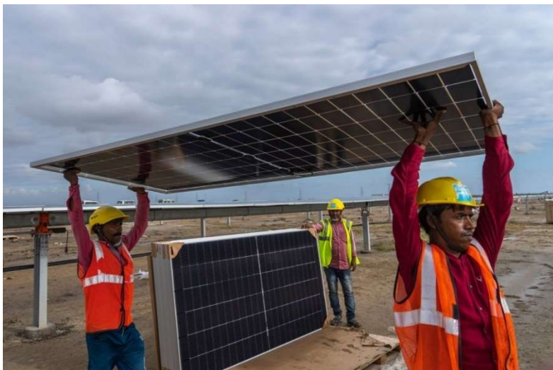
Installing solar panels at Adani Green Energy's Renewable Energy Park in India. Photo: Rafiq Maqbool/Associated Press
