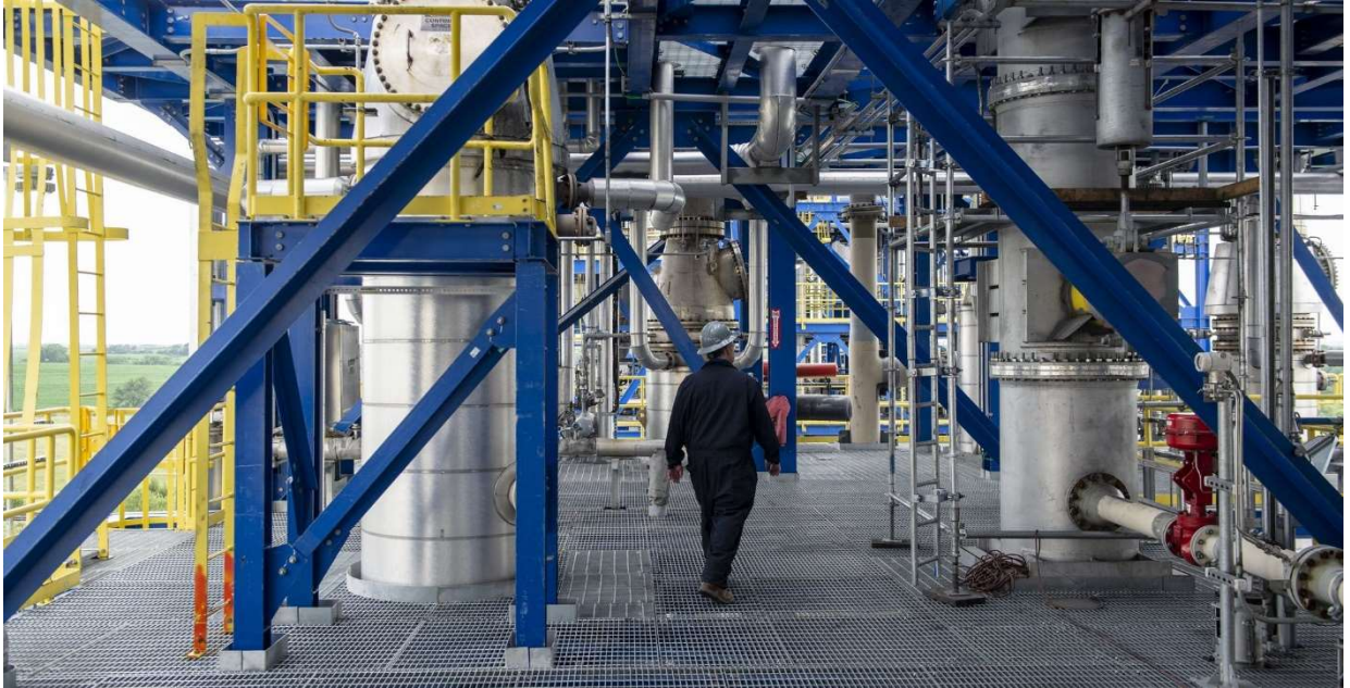
Hydrogen production is seen as a viable fossil-fuel replacement for heavy industry, unlike many other renewable-energy sources. The image shows Monolith's plant in Nebraska runs on renewable power to turn natural gas into clean hydrogen and carbon materials. Image credit: The Wall Street Journal
