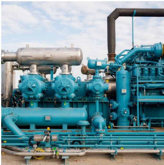
BKV compressor units process carbon dioxide in Bridgeport, Texas, before it is injected into a well. Denver-based BKV says that by the 2030s it will store millions of tons of climate-warming carbon dioxide in wells deep underground to eliminate or offset all the emissions generated from manufacturing and using its gas. Image credit: The Wall Street Journal.
